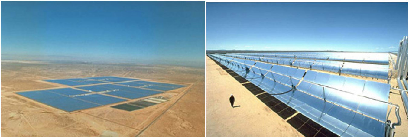
Concentrated solar power (CSP) plant in the Mojave desert, California, USA
