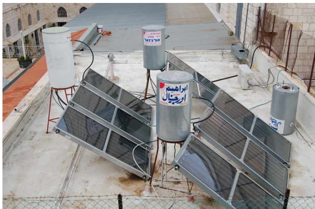
Solar water heaters on the roof of a house in Jerusalem
